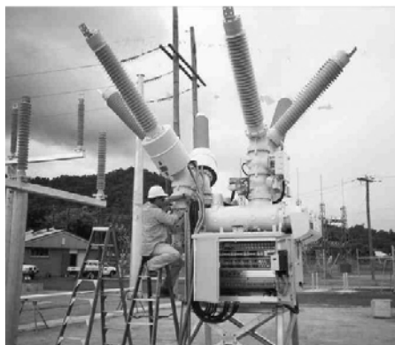
B65 Hybrid 145 kV in Australia
