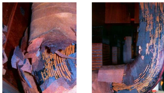
Figure 7: Connection of LV winding to LV bushing at a 181 MVA generator step-up transformer with obvious signs of pyrolysis
