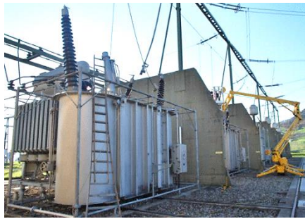
Figure 8: 220/150 kV and 140 MVA single phase transformer
