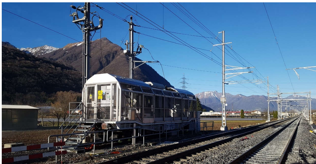
Abbildung 8: Mobiler Autotransformator SBB (ATmob) in Contone
