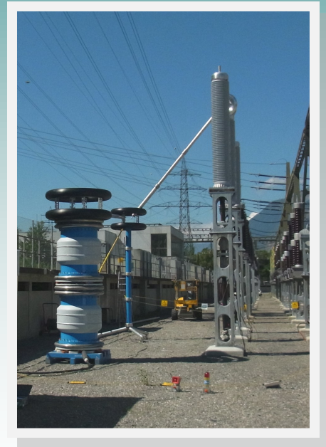
High-voltage resonance test on a 275 kV cable connection
