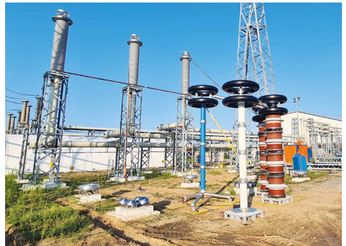
Figure 8: High-voltage test system for a 420 kV GIS test (voltage via an outdoor bushing)
