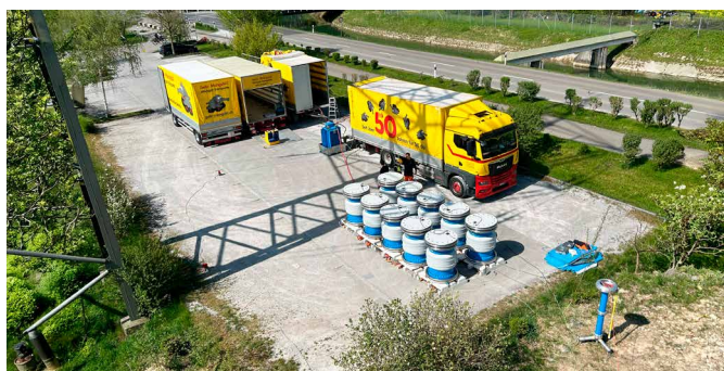
Figure 5: Series resonance system for cable testing without partial discharge measurement
