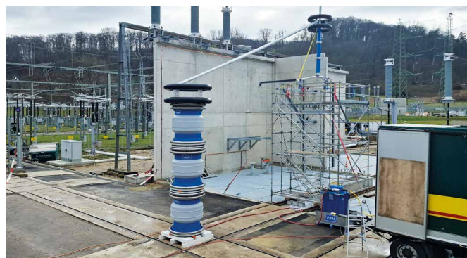
Figure 6: Resonance testing system for a 220 kV cable system with partial discharge measurement
