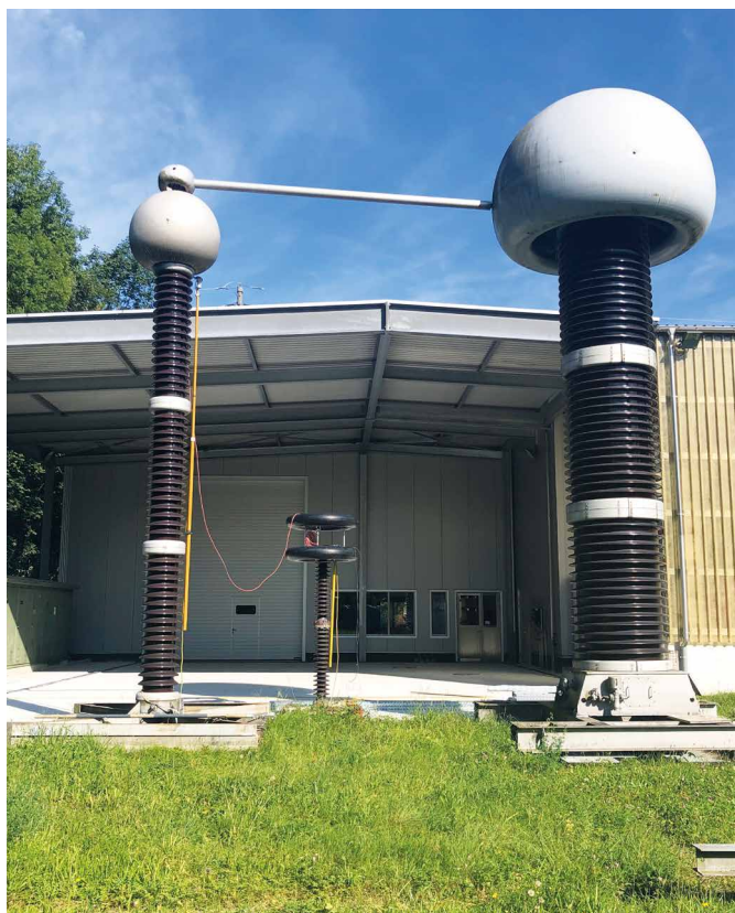
Figure 27: 1 MV test transformer manufactured by Moser Glaser AG
