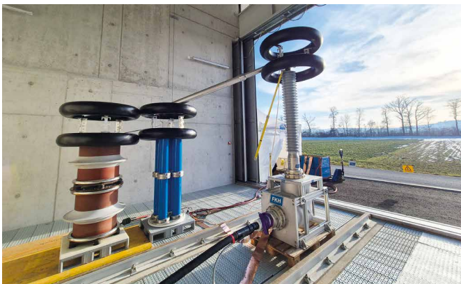
Figure 7: High-voltage test system for a 145 kV GIS test (voltage via Connex test cable, size 6)
