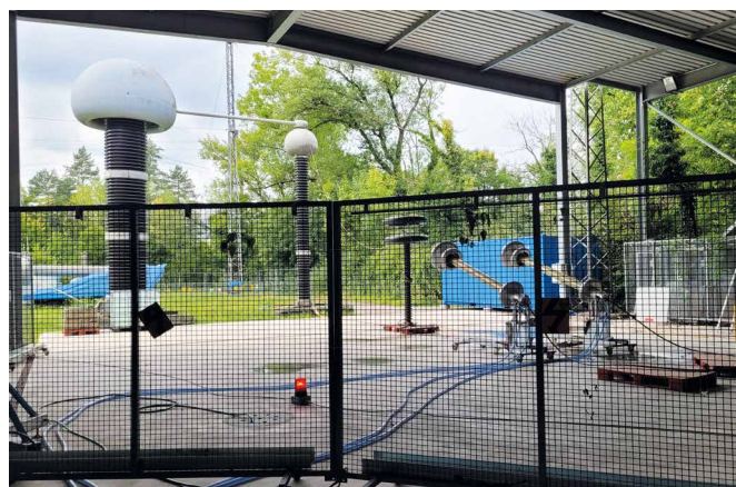
Figure 30: Covered forecourt of the test hall with a test rig for step tests, powered by the 1 MV test transformer (in the background)
