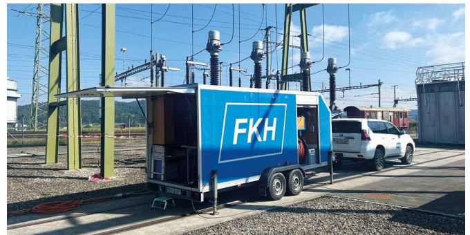
Figure 12: Mobile source for generating the experimental earth fault current
