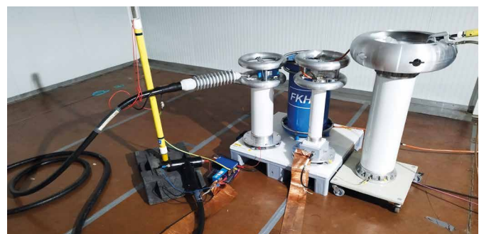
Figure 26: Testing a test cable using a series resonance system in the small laboratory (from left: test cable, coupling capacitor, resonance reactor, voltage divider and additional load capacitor)
