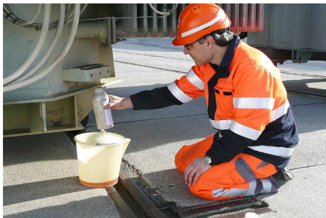
Figure 20: Oil sampling from a transformer
