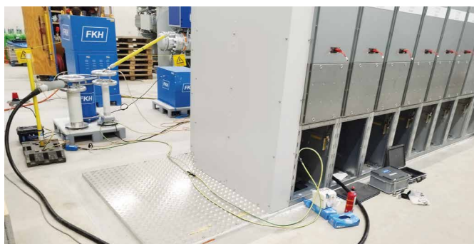
Figure 9: Testing of a medium-voltage switchgear
